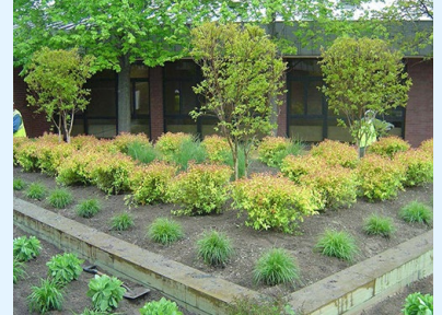
Green infrastructure elements such as planter boxes were incorporated into cleanup at the Curtis Bay Coast Guard Yard in Baltimore, Maryland. The tiered planting system filters stormwater and reduces stormwater runoff entering the sewer system. 21
