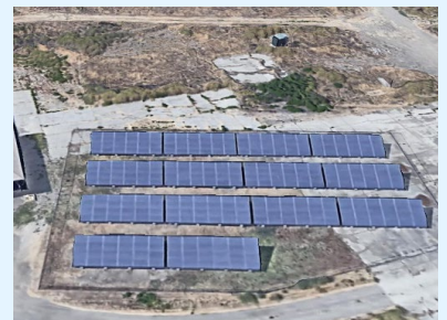
Optimization of a P&T system operating at the Frontier Fertilizer Superfund site in Davis, California, since 1995 has included energy efficiency measures such as:
