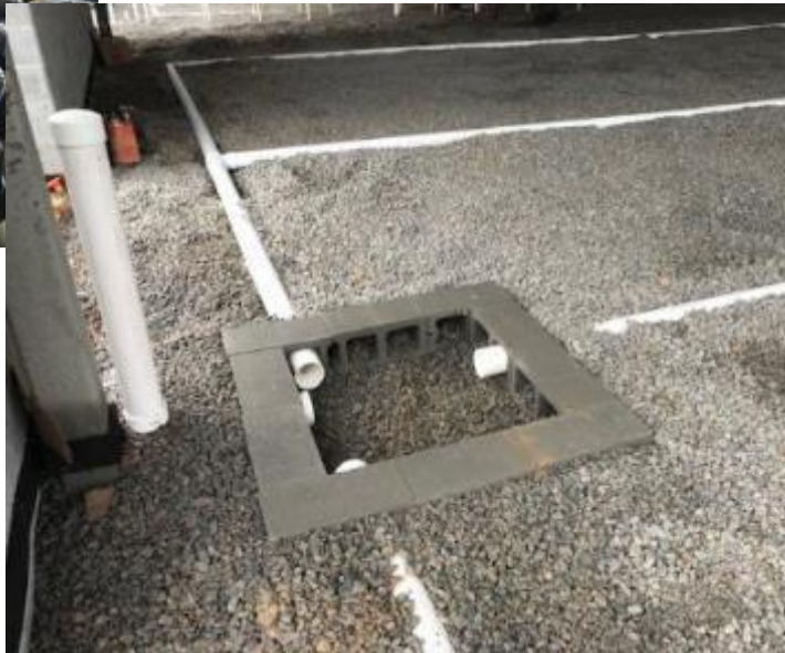
Passive Sub-Slab Venting (SSV) Systems
