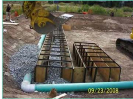
Construction of the BCR in Park City, UT Photo courtesy Jeff Schoenbacher Park City Municipal Corporation
