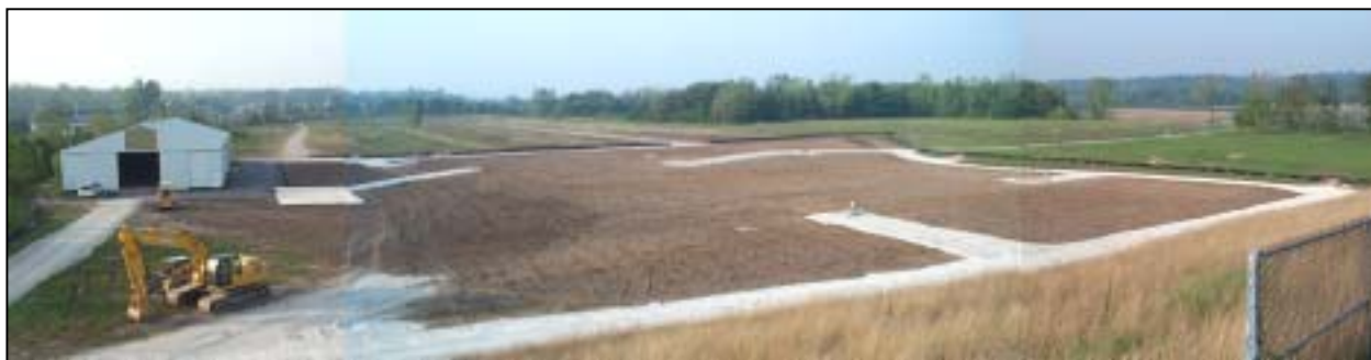
Figure 5-7. A newly completed AFC over a RCRA solid waste management unit in Missouri.
