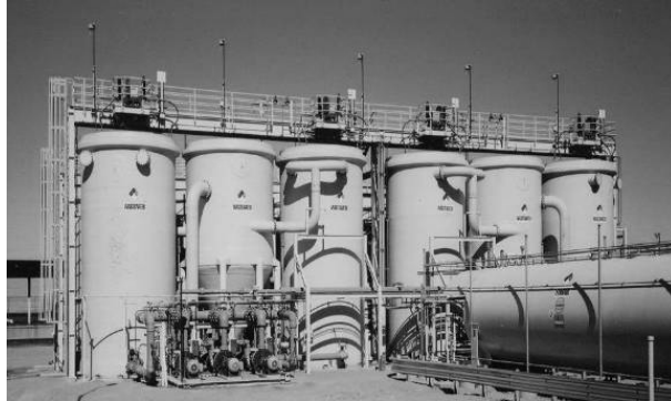
Fluidized Bed Reactor (FBR) System in Henderson, Nevada
