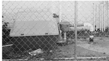
Figure 6-1. Small-scale soil vapor extraction (SVE) system designed to address the source of vapors. Photo Source: Vapor Mitigation Sciences, LLC.
