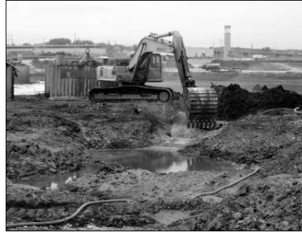
Excavator bucket mixing of contaminated sediment of a former steel mill operation, Sydney Tar Ponds, Sydney, NS, Canada.
