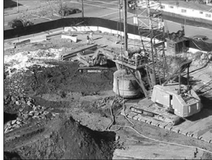
Auger-mixed in situ S/S treatment of a former manufactured gas plant (MGP) site with coal tar contaminants at Kendall Square, Cambridge, MA, United States.
