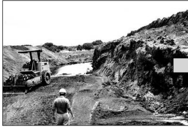
Battery Recycling Site
