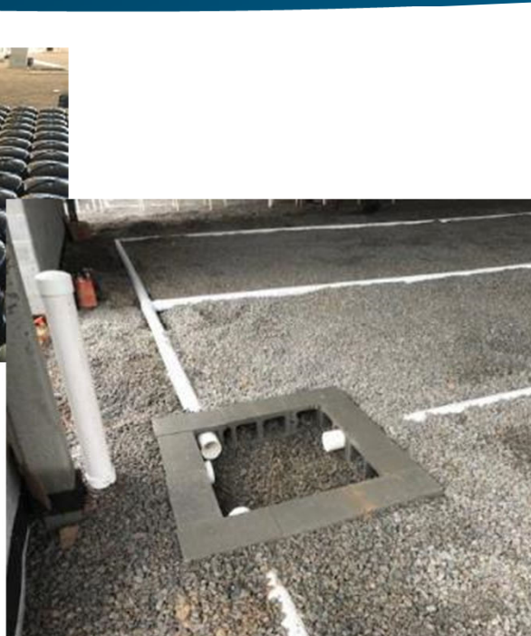
Passive Sub-Slab Venting (SSV) Systems
