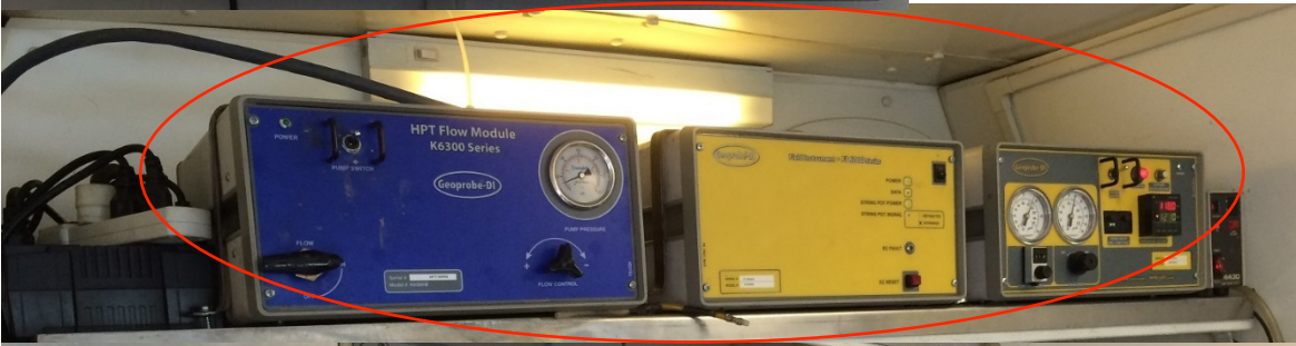
Trunk line controls
