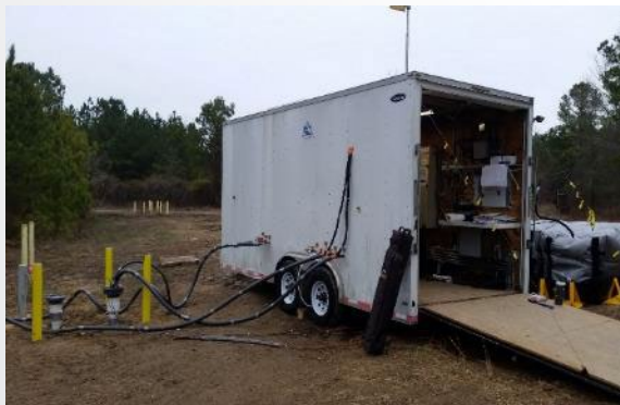
EK Pilot Test System Trailer
