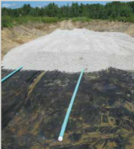
Limestone is added to a vertical flow pond during construction of a passive treatment system to treat AMD in the South Fork Tangascootack Creek.
