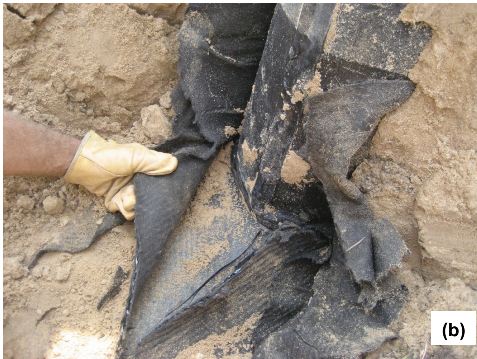
Fig. M. 14. Examples of seams observed during exhumation: (a) dual-track wedge weld and (b) extrusion well to boot for gas well near Test Pit 4.
