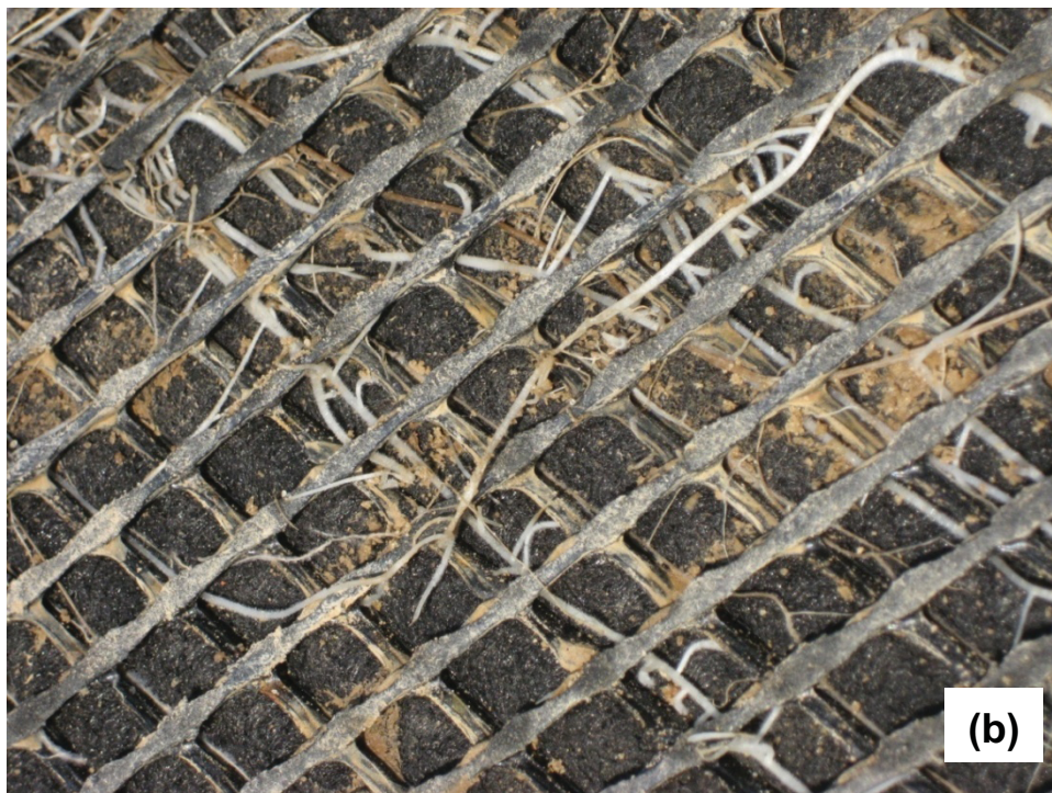
Fig. M. 13. Roots in the GDL and fines coating the ribs of the geonet in Test Pit 1: (a) overview and (b) close up.
