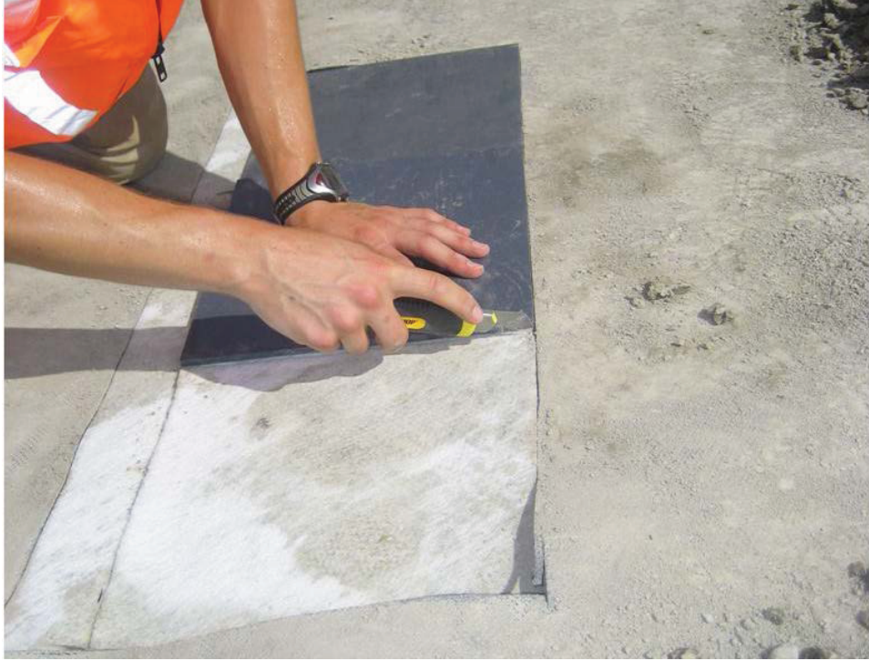
Fig. M. 21. Cutting of GCL sample perimeters in Test Pit 2. Staining visible on GCL carrier geotextiles.
