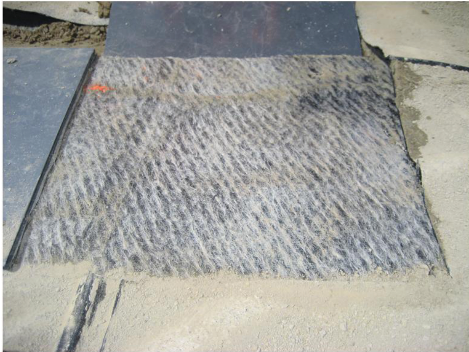
Fig. M. 23. Moisture visible on GCL after rupturing GM patch in Test Pit 1.
