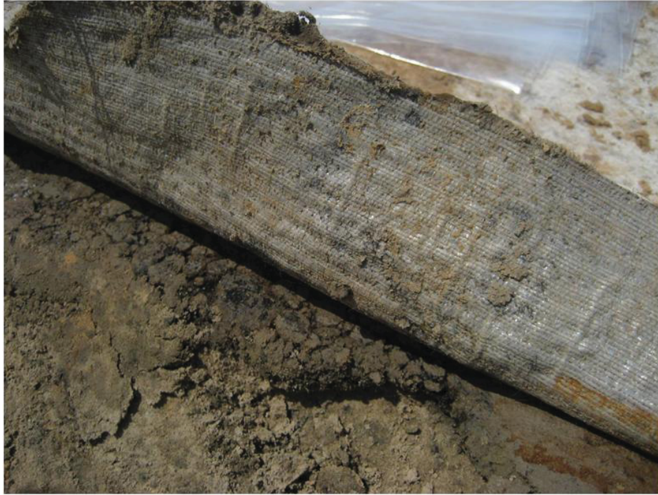
Fig. M. 18. Black and rust colored staining underlying Site E GCL.
