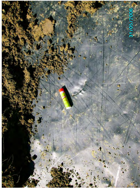
Fig. A.52. Unintentional hole from installation found via geophysical investigation.
