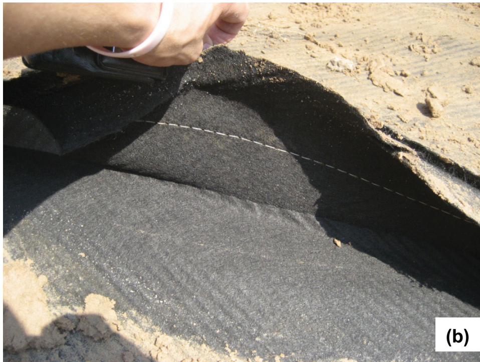
Fig. M. 12. Seam joining geotextiles in adjacent GDL panels in: (a) seam after removing cover soil (fish mouth in middle is due to disturbance during excavation) and (b) close up showing stitching of geotextiles and clean geotextiles in the overlap.
