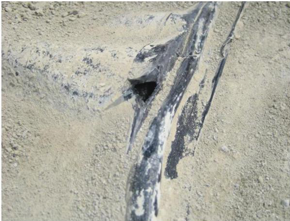
Fig. M. 24. Puncture visible in GCM patch weld in Test Pit 1.
