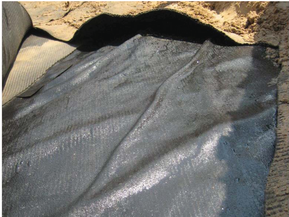
Fig. M. 11. Moisture visible across GM immediately after GDL removal.
