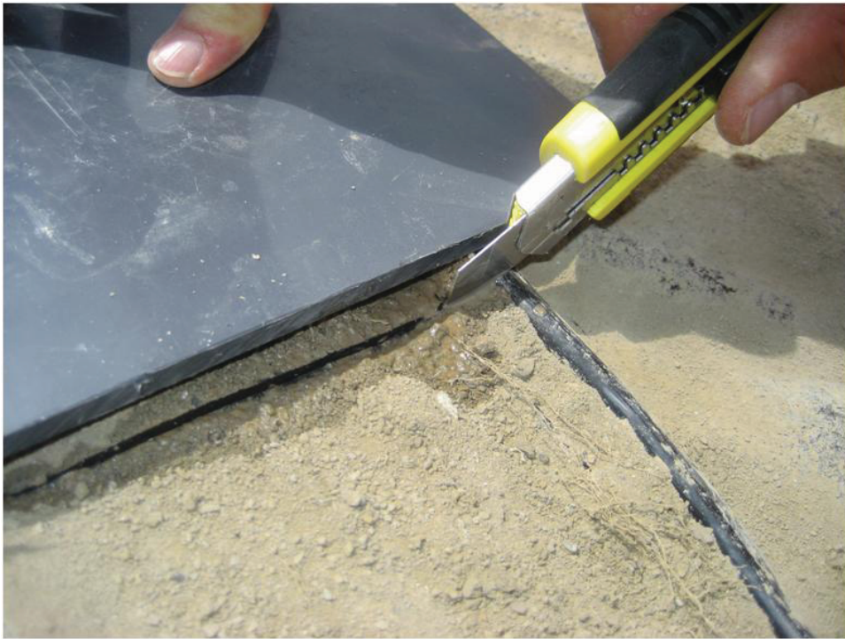
Fig. M. 22. Moisture seeping from GM while cutting through GM patch in Test Pit 1.
