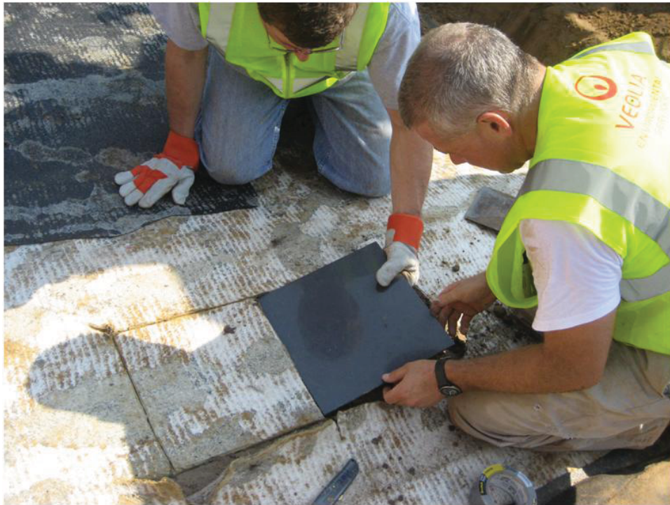
Fig. M. 17. GCL sample with cut perimeter prior to sliding of sampling plate and removal.
