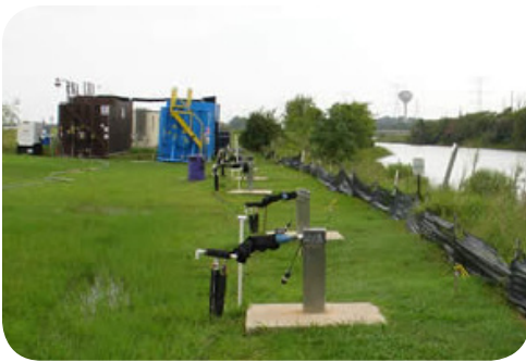
Groundwater Pumping Wells
