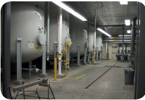
Indoor Treatment Facility
