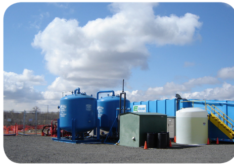
Outdoor Treatment Facility
