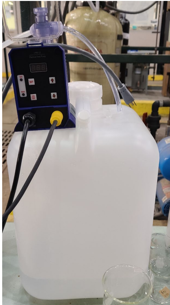
Figure 4. Hydrogen peroxide injection system
