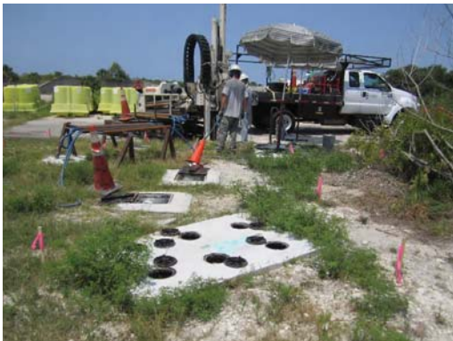
Well box locations in the injection area
