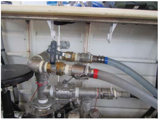
Transfer Line Manifold on top of Progressive Cavity Pump
