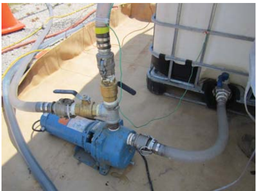
Transfer Pump bonding location
