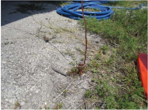
Copper spike for injection rig grounding wire
