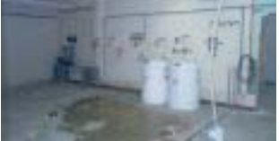
Figure 7: Photo of recirculation system at PIA
