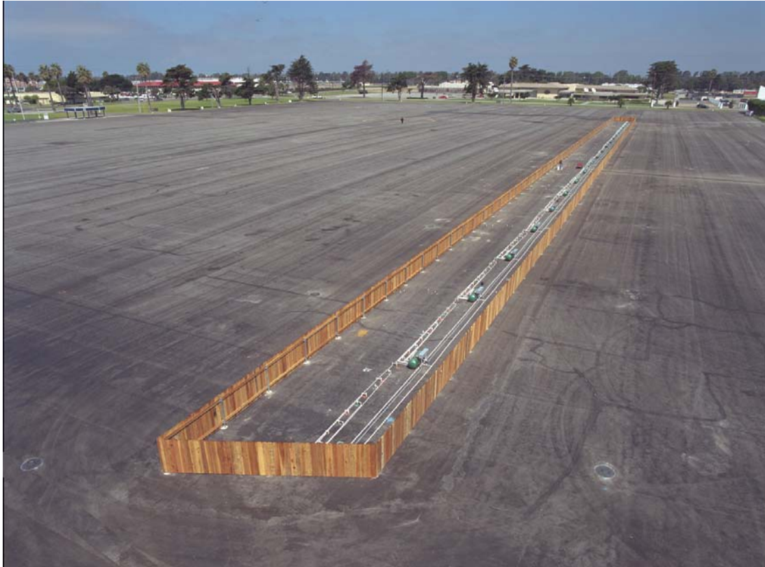
Figure 3-1. Large-scale Biobarrier PTB System at NBVC (Port Hueneme, California). The Fenced-in Area is Approximately 600-ft Long.
