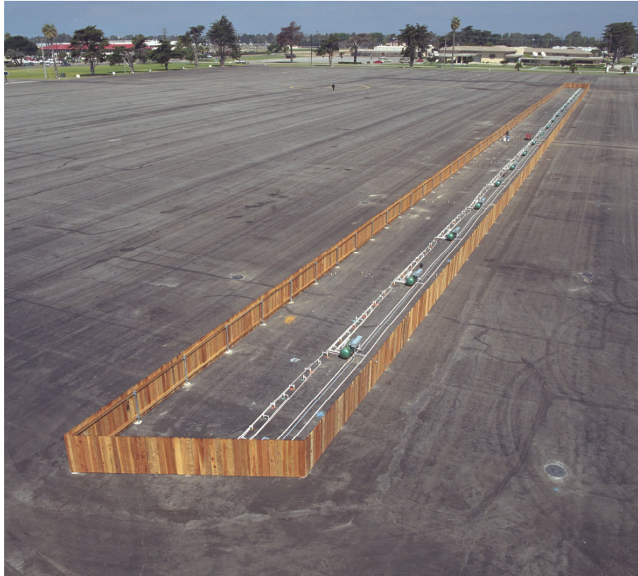
Figure 2. Full-scale biobarrier located at NBVC, Port Hueneme, California (groundwater flows from right to left).
