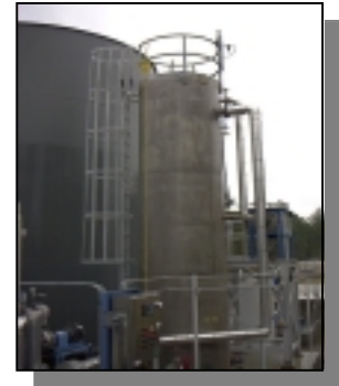
Fluidized Bed Reactor (FBR) at LHAAP
