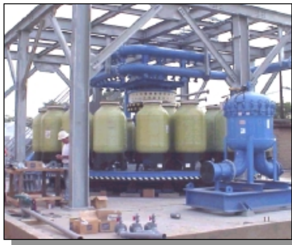
La Puente, California, Ion Exchange System
