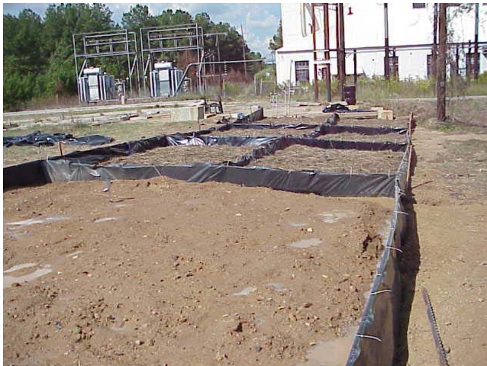
Figure 7. Photographic view of the pilot scale test layout immediately after addition of the liquid amendments.
