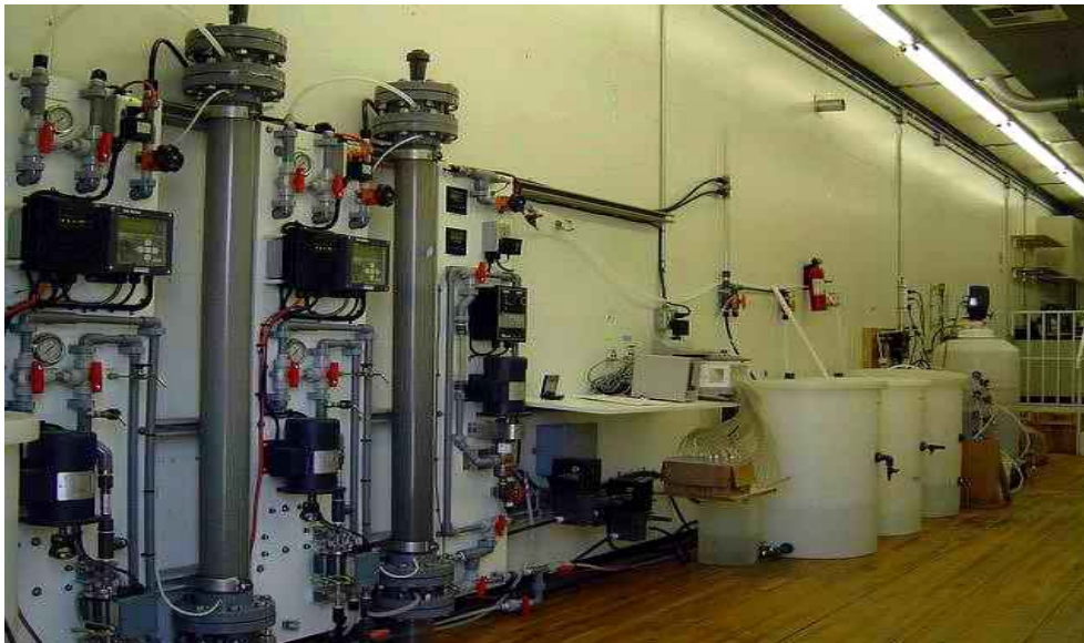
Figure 4-2. IX with brine treatment pilot plant.
