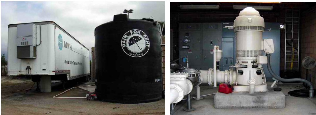
Figure 4-1. Pilot plant trailer, influent reservoir, and well pump head.
