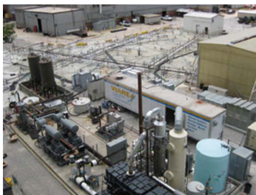
Figure 3. Completed IST system covering approximately 27,400 square feet of industrial space at Arnold Air Force Base.
