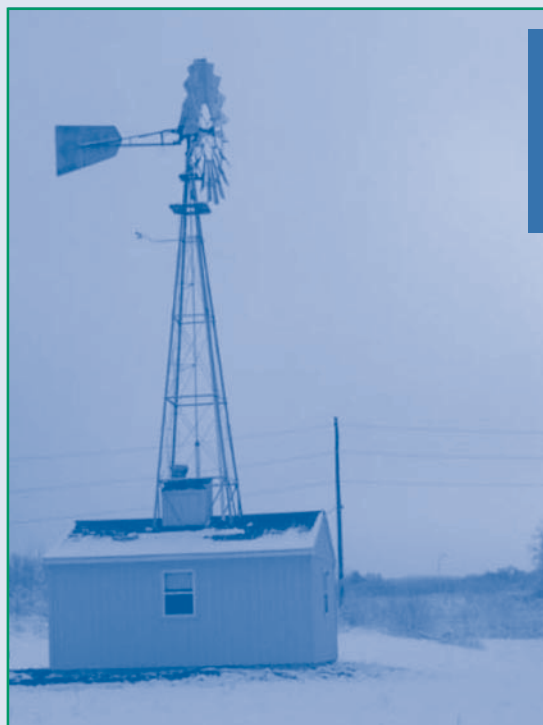
Figure 1. Ferdula landfill gas extracted by wind-generated vacuum is treated inside a 150-ft 2 building co-located with the windmill.
