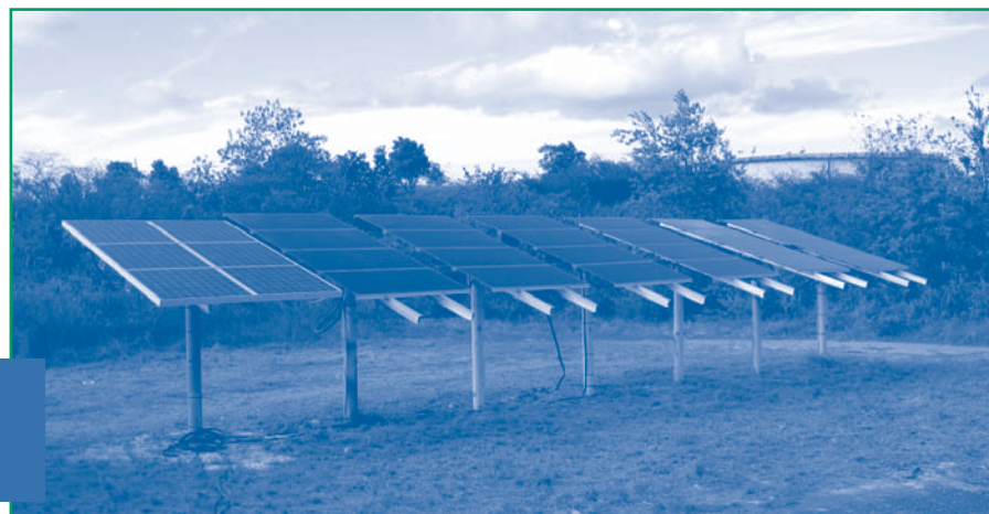
Figure 2. The SCA solar system for fluid gathering now consists of a 385-W PV array in fixed-tilt position.
