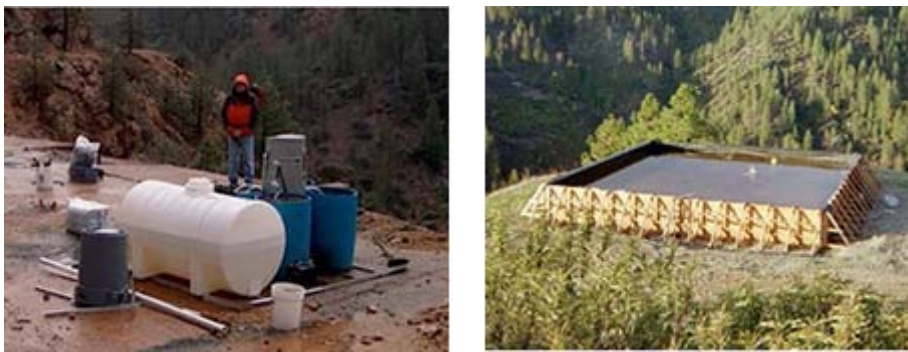
Figure 3. Bench-scale testing (left) and pilot-scale application of a BCR treating ARD at a rate of approximately 1 gpm (right) at the Golinsky Mine
