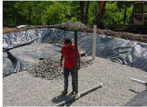
Figure 2. Limestone emplaced in three lined, underground treatment cells at the Kimble Creek site
