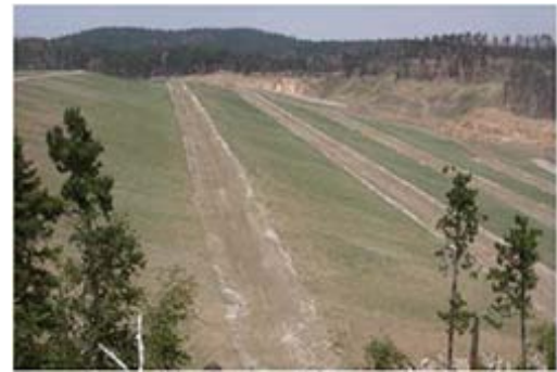
Figure 6. Five uppermost slopes and drainage channels along the capped Ruby Gulch waste repository, approximately three months after seeding
