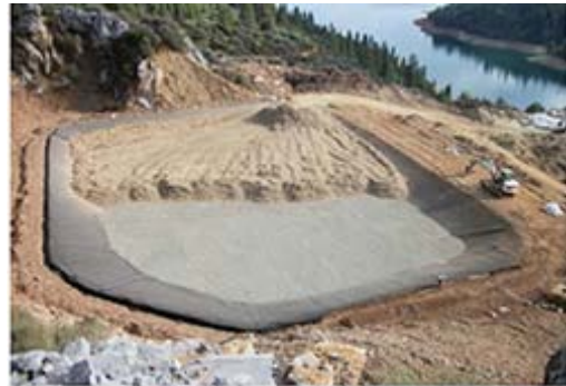
Figure 6. Placement of media in the Golinsky Mine BCR
