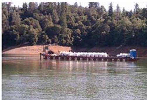
Figure 4. Barge delivery of sacks filled with organic media or other construction materials such as drainage gravel and rip rap needed for the Golinsky Mine BCR
