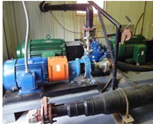
Figure 4. The Strawberry Creek pumping station, one of three primary facilities for water management at the Gilt Edge Mine
