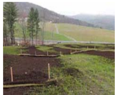
Figure 5. Slope stabilization and erosion control at the Elizabeth Mine Superfund Site was achieved using a compost blanket combined with tubular sediment control devices.
