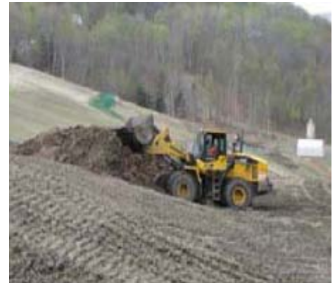
Figure 4. Organic-rich topsoil for the 45-acre cap at Elizabeth Mine Superfund Site was manufactured onsite.
