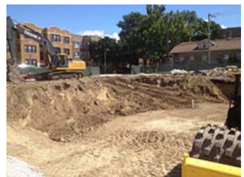
Figure 4. Diesel equipment such as a 250-horsepower excavator and 100-horsepower soil compacting roller operated under an idle restriction plan at the Whitney Young Library site.
