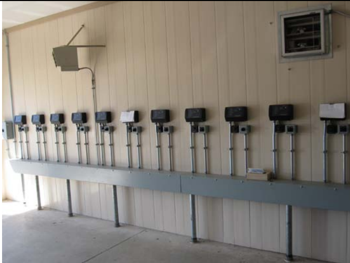
3 HCS Building Interior – Well Pump Controls.
