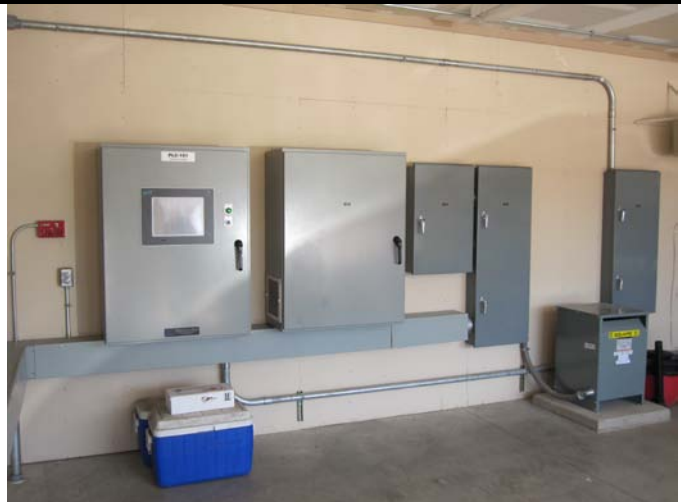
6 HCS Building Interior – Electric and Control Panels.
