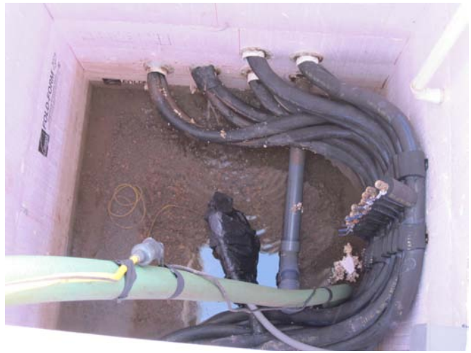
2 HCS Recovery Well Vault Interior. Note: Double-Contained Separate Lines to Each Well.
