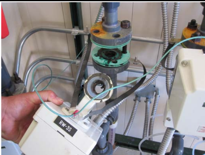
5 Closeup of Well Piping and Flow Meter Maintenance.
