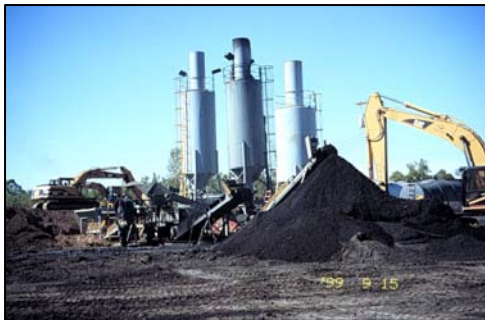
Figure 7-1. Ex-Situ Treatment at ACW
