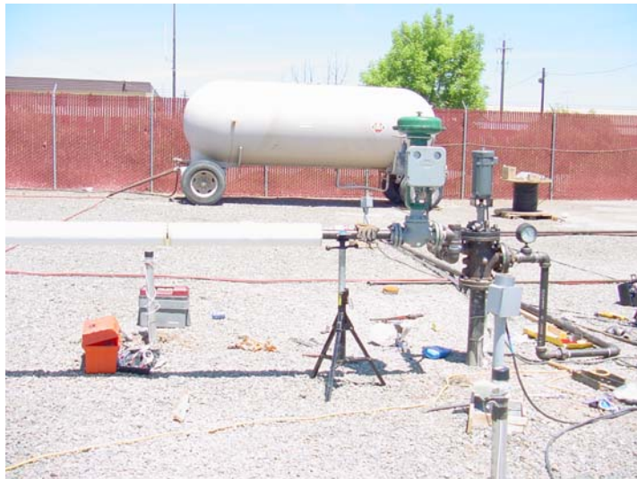
(a) 5,500-gal Propane Gas tank
