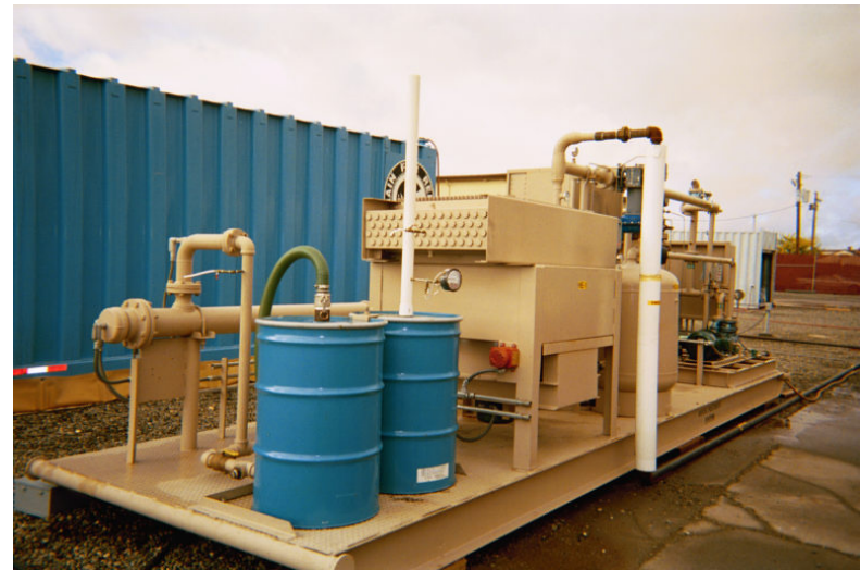
(c) Vapor-Extraction Treatment System
