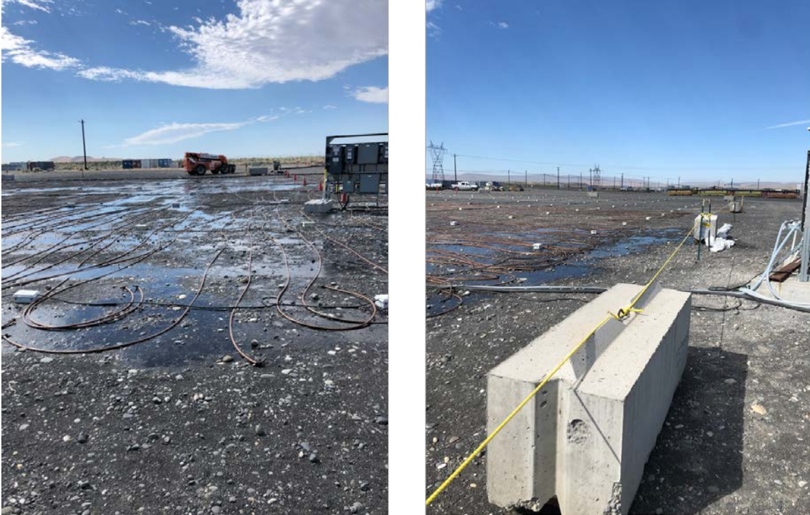
Figure 6. (left) Photograph taken during the first week of soil flushing in 2022, highlighting flush water distribution lines. (right) Photograph highlighting the ERT electrode array (white boxes connected by cables)
