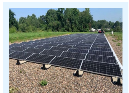
At the 42-acre Solvents Recovery Service of New England site in Connecticut, a 53 kilowatt PV system directly powers pumps that extract contaminated groundwater. An infiltration gallery and green infrastructure such as vegetated swales help manage the site’s stormwater and prevent onsite erosion. Remy design and construction considered the site’s anticipated use as an open-space area. Plantings of approximately 2,700 native trees and shrubs helped restore onsite biodiversity and wildlife habitat while alleviating flooding along banks of the bordering Quinnipiac River. 2
