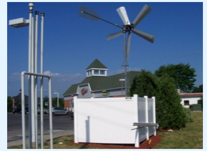
A mechanical windmill directly powered the compressor required for biosparging at an underground storage tank site. 8
