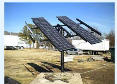
A 560 watt passive PV system provided power to extract contaminated groundwater for ex situ treatment at the Busy Bee's Laundry in Rolla, Missouri. The PV system was scaled to meet the expected energy demand of one 400-watt surface-mounted piston pump, which was rated at 9.1 gallons per minute at 140 feet of total dynamic head. Use of the PVWatts tool estimated a potential pumping period of 55 to 89 hours per month. The PV system included a passive tracking mechanism to maximize solar energy capture throughout the day. 13
