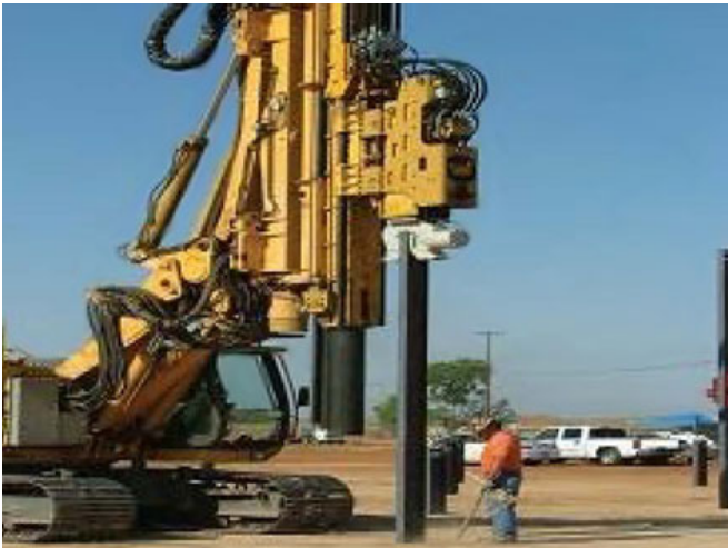
PV Mount Installation: A vibratory hammer was used to press vertical beams needed as solar module mounts into the ground, which minimized earth moving and soil disturbance.
