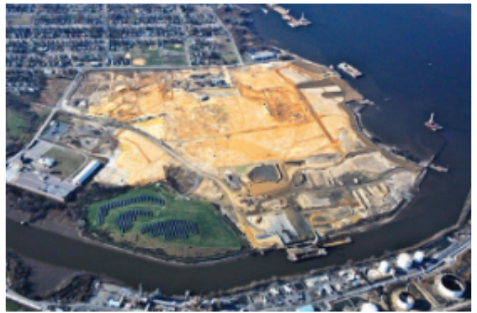
Current Infrastructure Port: All planned remediation systems began operating by the end of 2012. The deep-water port is anticipated to begin accepting ships in 2015.
