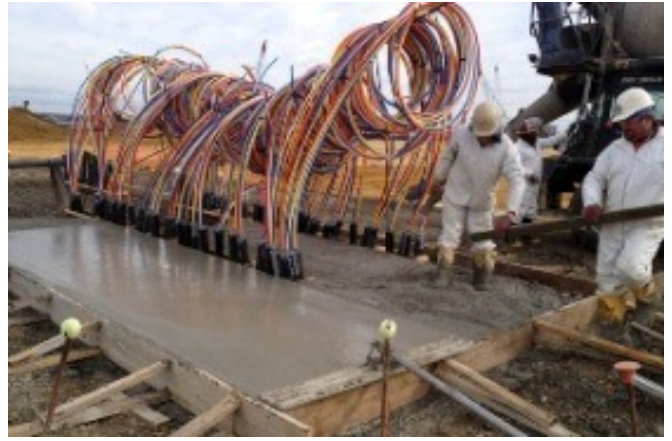
Ozone Sparge System Installation: In 2011, an ozone sparge system was installed to accelerate removal of contaminant vapors from groundwater in two contaminant source areas.
