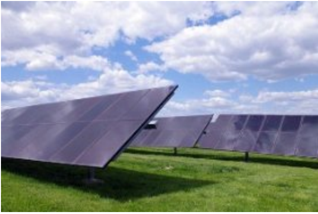
PV Arrays: Each PV array was installed on concrete footers designed to accommodate the landfill cover system's operation and maintenance requirements.
