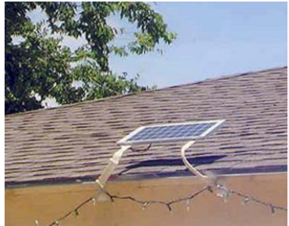
Each solar panel is installed at a 25-50° tilt with unobstructed southern exposure to the sun.
