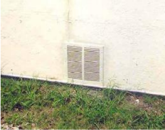
Each crawl space exhaust system vents to the building's exterior at ground level.
