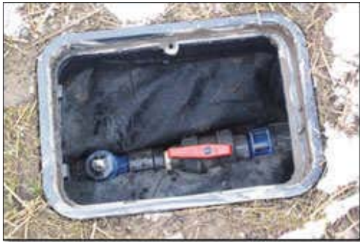
A subsurface valve box at each gas vent is used to control vacuum throughout the landfill and for sampling purposes.
