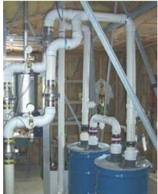
Check valves were installed on each side of the air cylinder so a vacuum could be generated during both the up and down strokes of the windmill.
