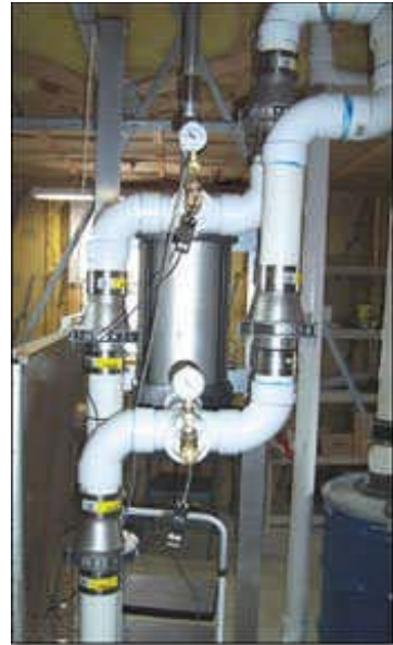
Check valves were installed on each side of the air cylinder so a vacuum could be generated during both the up and down strokes of the windmill.
