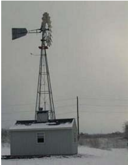
Landfill gas extracted by the windgenerated vacuum system is treated inside an adjacent 150-ft 2 building.
