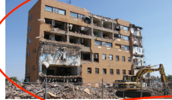
Buildings with asbestos and lead paint
