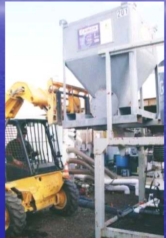
Loading Permanganate Storage Hopper
