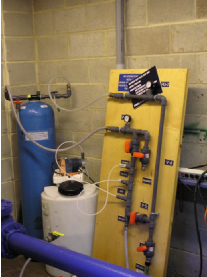
Figure 2-3. ADI International Inc. Pilot Test Unit. No. 2002-09 with Media G2 ® as installed at the HTWSA Well Station No. 1.
