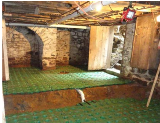
Figure 5. Slab construction using a synthetic base layer into which concrete was poured for homes with basements having dirt floors.
