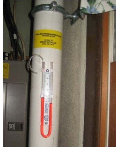
Figure 3. Interior plumbing of the typical sub-slab depressurization systems, including a U-tube manometer providing real-time measurements.
