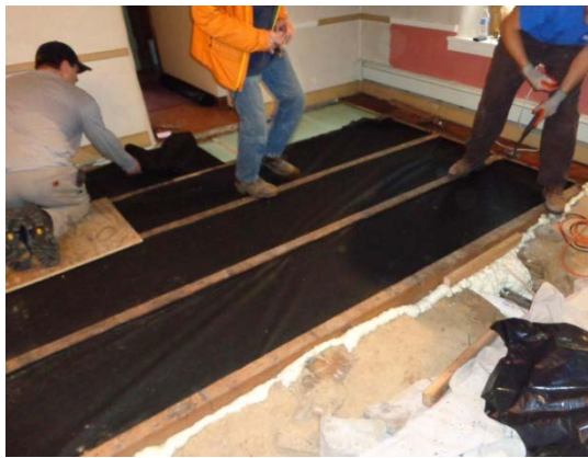
Figure 4. Installation of high-density polyethylene sheets serving as vapor barriers in several homes near the Crossley Farm site.
