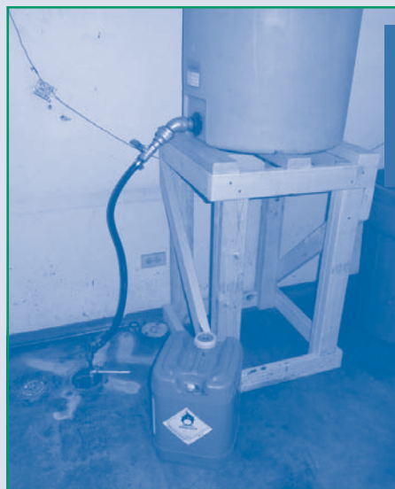
Figure 3. ISCO at the Norgetown Cleaners relied on six gravity-feed lines of various lengths to reach 32 injection points inside or directly outside the drycleaner building.
