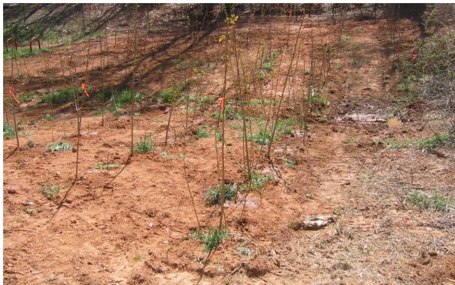
Figure 5. 04/05/06. View of site looking east across drainage area. Note seepage area.
