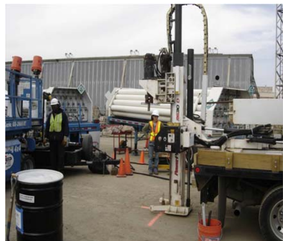
Figure 3-3. PFI Pneumatic Injection Equipment Layout
