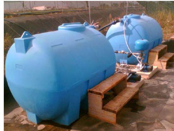
Tank for chemical additives
