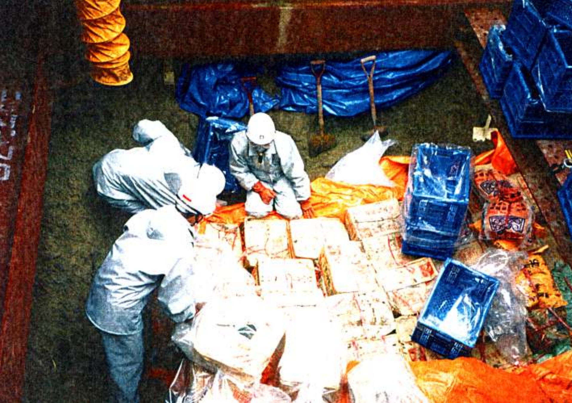
Pesticides were buried into sandy soil. The cardboard box including pesticides was wrapped by vinyl sheet. Because of effective waterproof with vinyl sheet contents of pesticides were in dry condition and identified.
