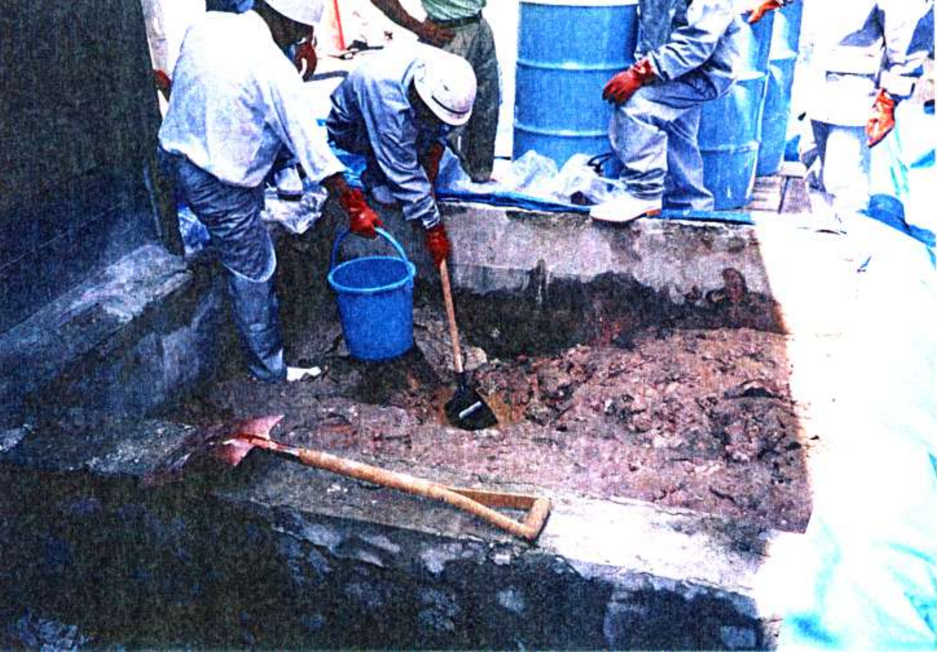
Pesticides were buried into a concrete frame. However, water entered and pesticides were soaked. It is a photograph after the supernatant is drained. What kinds of pesticides cannot be distinguished because these pesticides were soaked.
