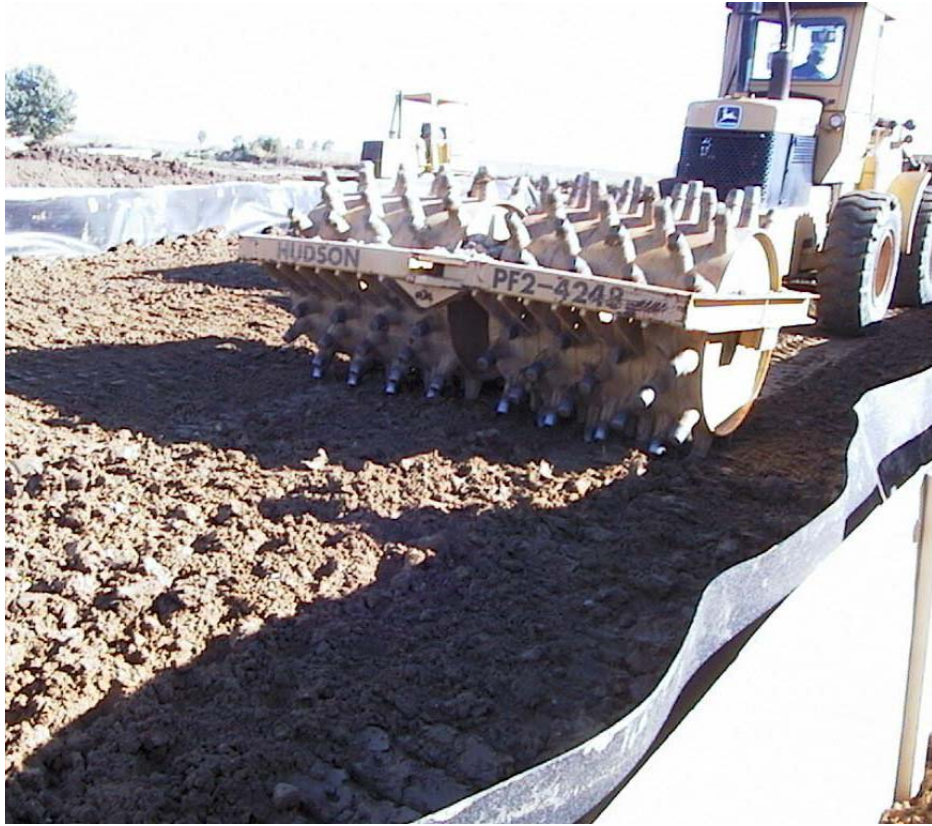
Tow-behind tamping foot compactor for clay barrier layer at Cedar Rapids site.
